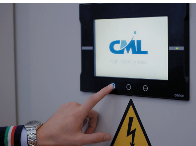
Operation terminal HMI NA series controls the complete line
