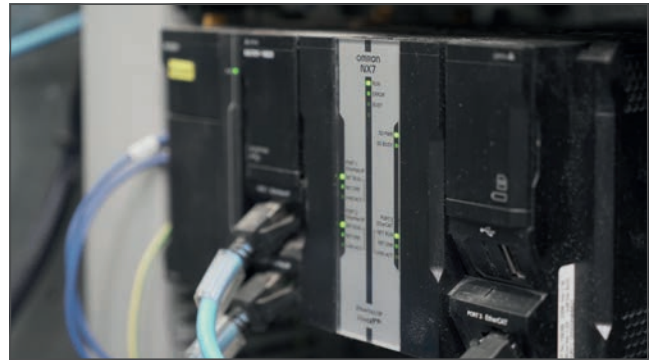
In addition to the five AMRs, OMRON also supplied the Sysmac machine controller.
