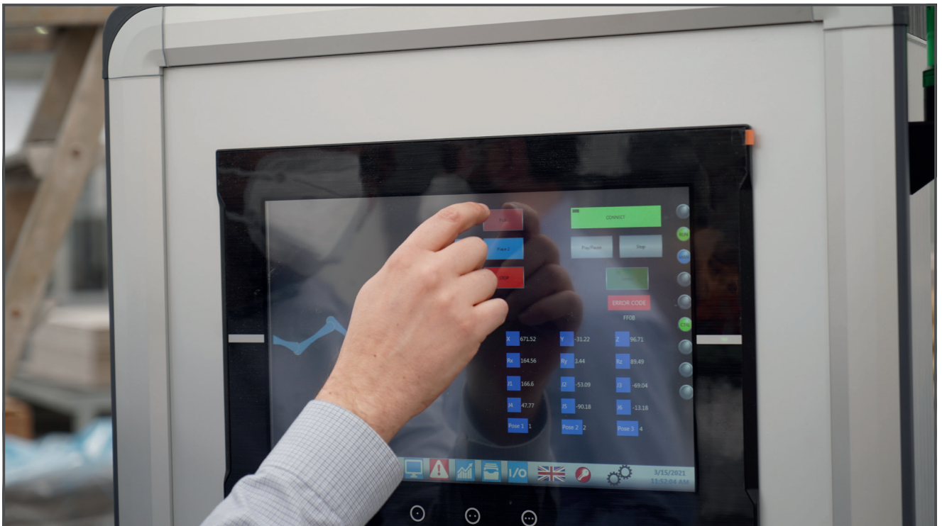
All of the data is sent to and managed centrally by an OMRON NX102 PLC, which is connected to the manufacturing execution system (MES).
