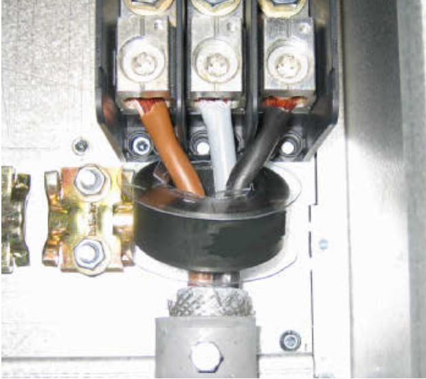
Fig. 55 Ferrite core mounted on the motor cables
