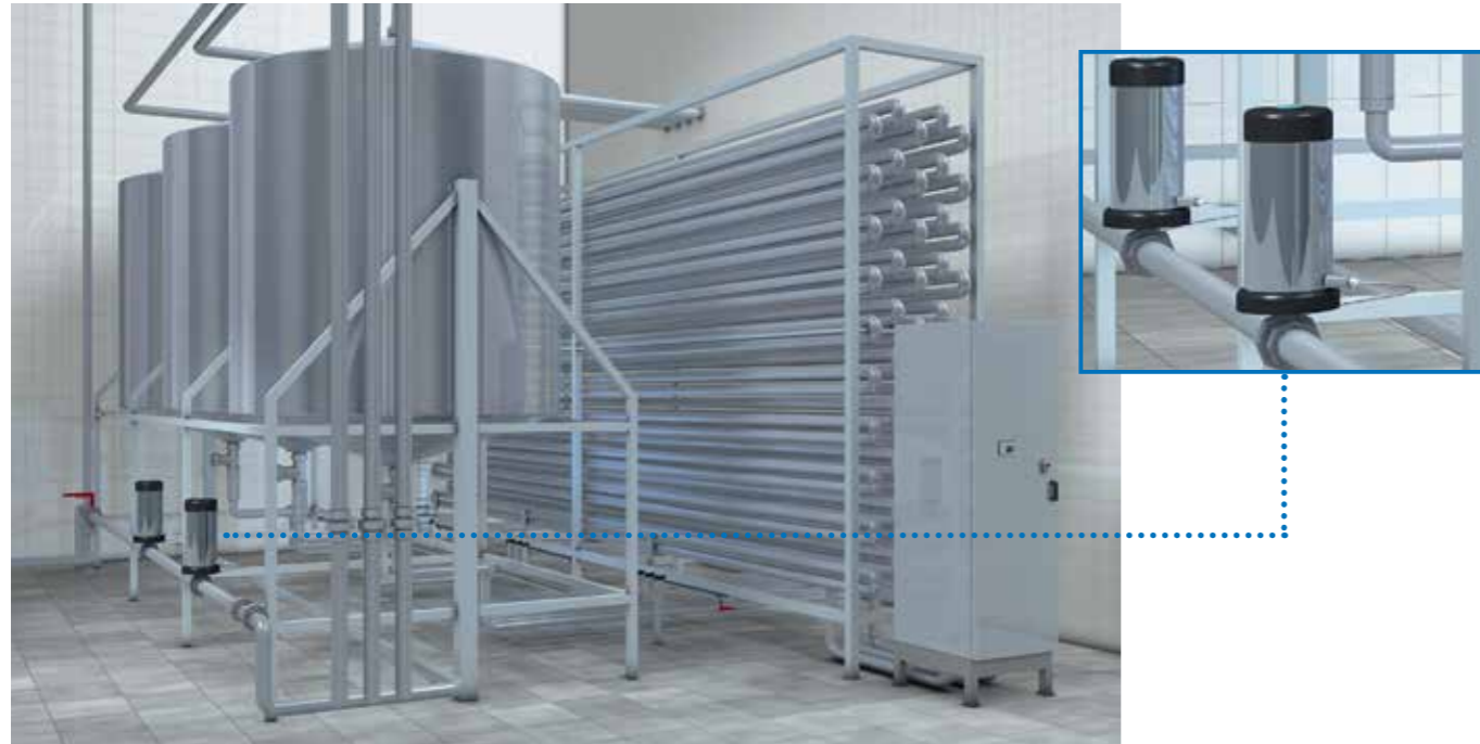
Control positioning of valves of the mixers or heating systems.
