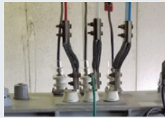
Abnormal heating of transformers caused by rise in ambient temperatures
