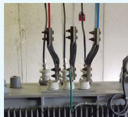
An abnormal exothermic of a transformer
